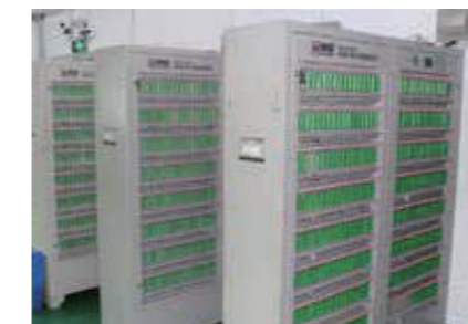
Battery Capacity Detection Cabinet
