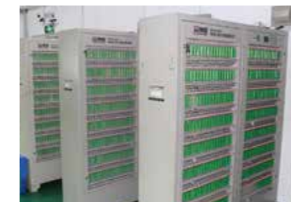
Battery Capacity Detection Cabinet
